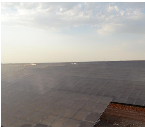
Photo: BELECTRIC Solar Power Plant Nataram near Mandasaur, India, with 23MW DC capacity.
