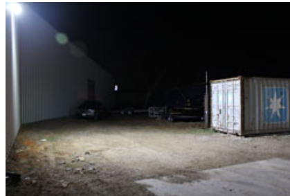
BLWP-60LED-36 mounted 15' high illuminating a 30' long by 50' wide parking area.
