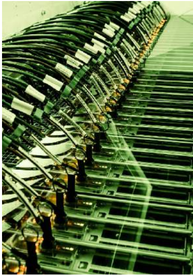
Fig. 5. The compute nodes submerged in the GRC Carnot Jet system
