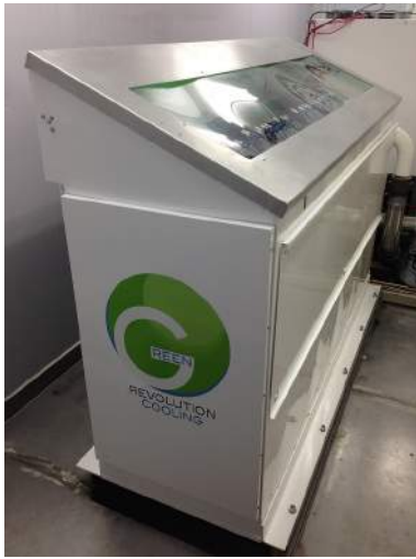
Fig. 4. The GRC Carnot Jet system installed inside the container
