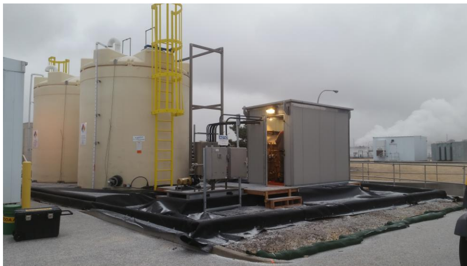
Metro Wastewater Reclamation District: North Plant PAA Storage & Delivery System
